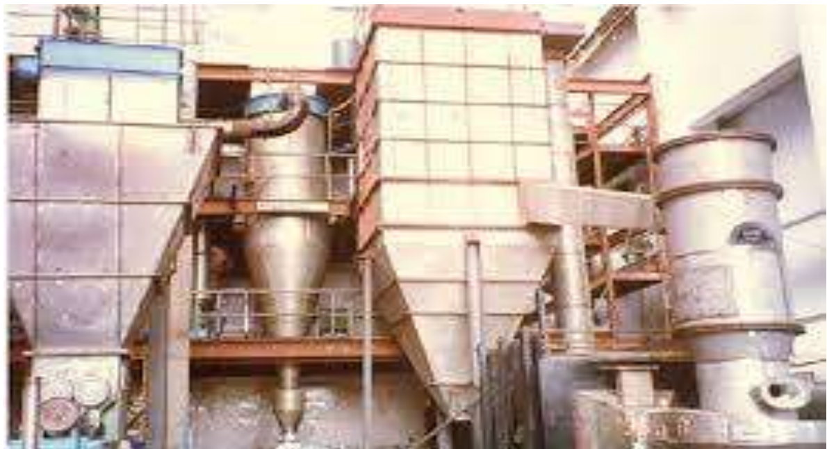
Process Plant at DTPL
